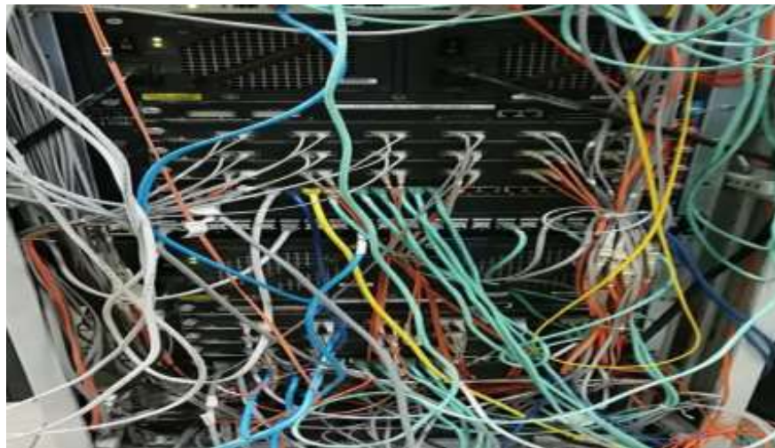
Figure 10. Old core switches
